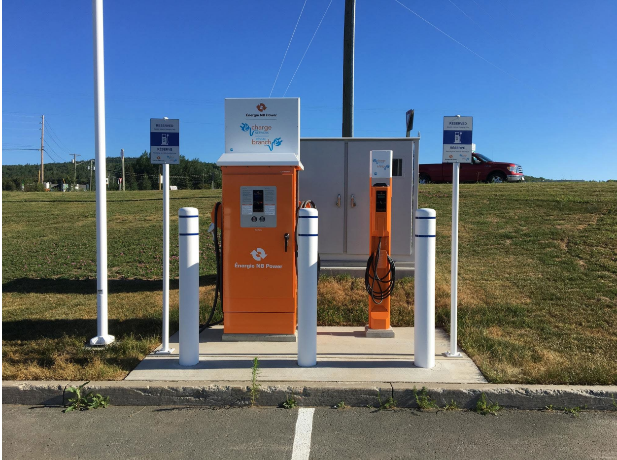
Figure 1: Image of an NB Power charging station with DC Fast charger (left side with two charging cords) and Level 2 charger (right side with one charging cord). Source: Osprey Truck Stop - DC Fast Electric Car Charging - 2 Martin, Eel River Bar, NB E8C 3C7, Canada - Gas Station - PlugShare
